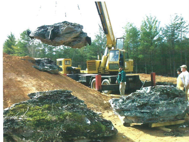
Work in progress. Those boulders the crew is placing weigh 10-11 tons each.
